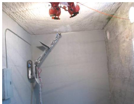
Remote sprayer platform applying fixative to hot cell mock-up facility at FIU Testing Facility.
